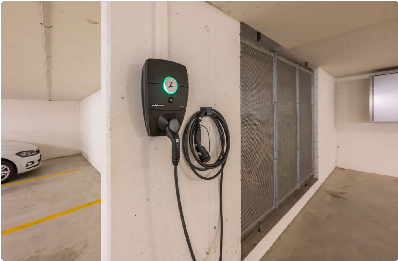
With e-car charging station
